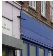
Colour disharmony between neighbouring units
