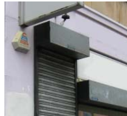
Canopy housing boxes protruding into the streetscape and not designed as part of the fascia
