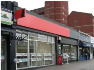
Facia signage does not relate to the location of columns
